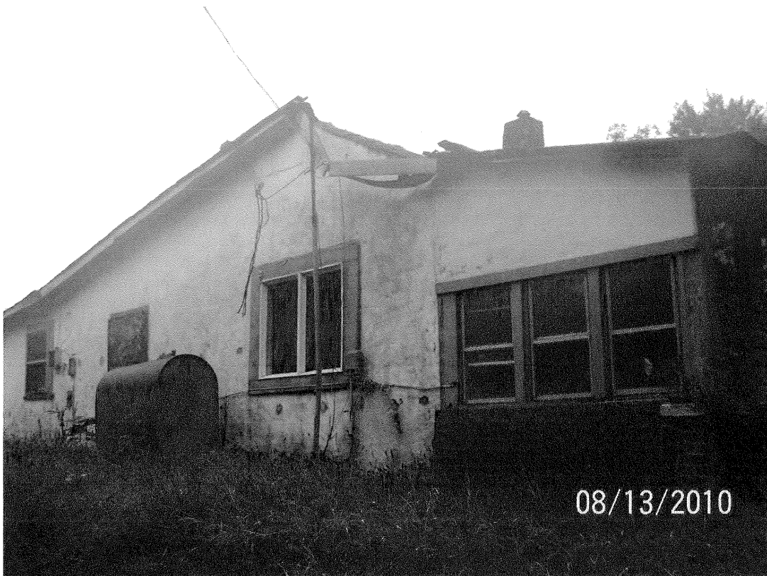
Side of structure shows damage to roof
