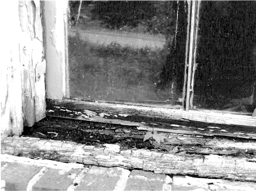
Wood trim deteriorated and exterior surfaces not weathertight
