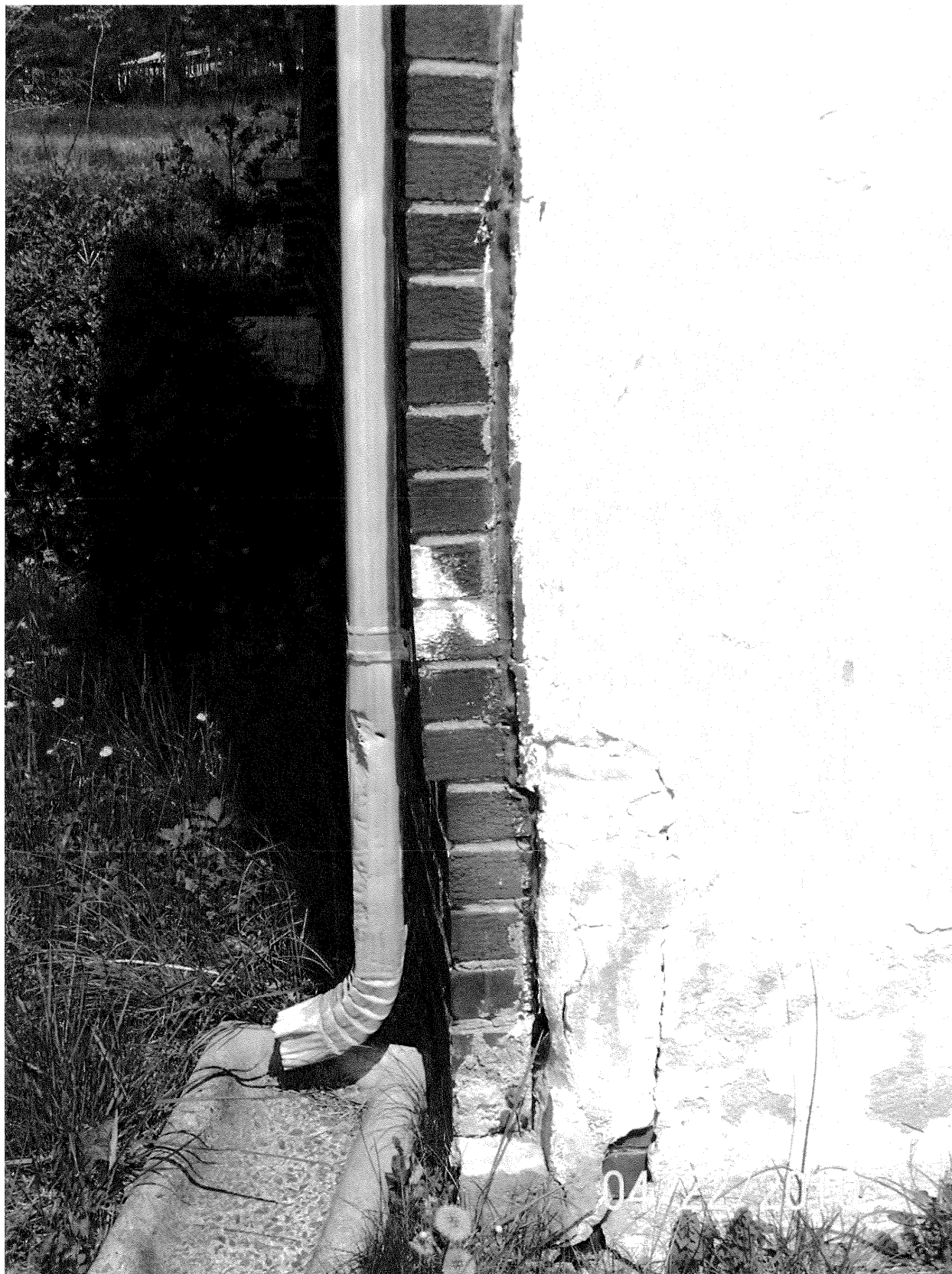
Walls and foundation of structure show evidence of shifting and racking
