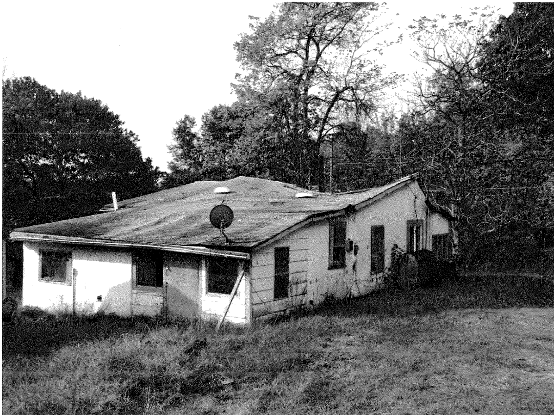
Rear of structure shows damage to roof
