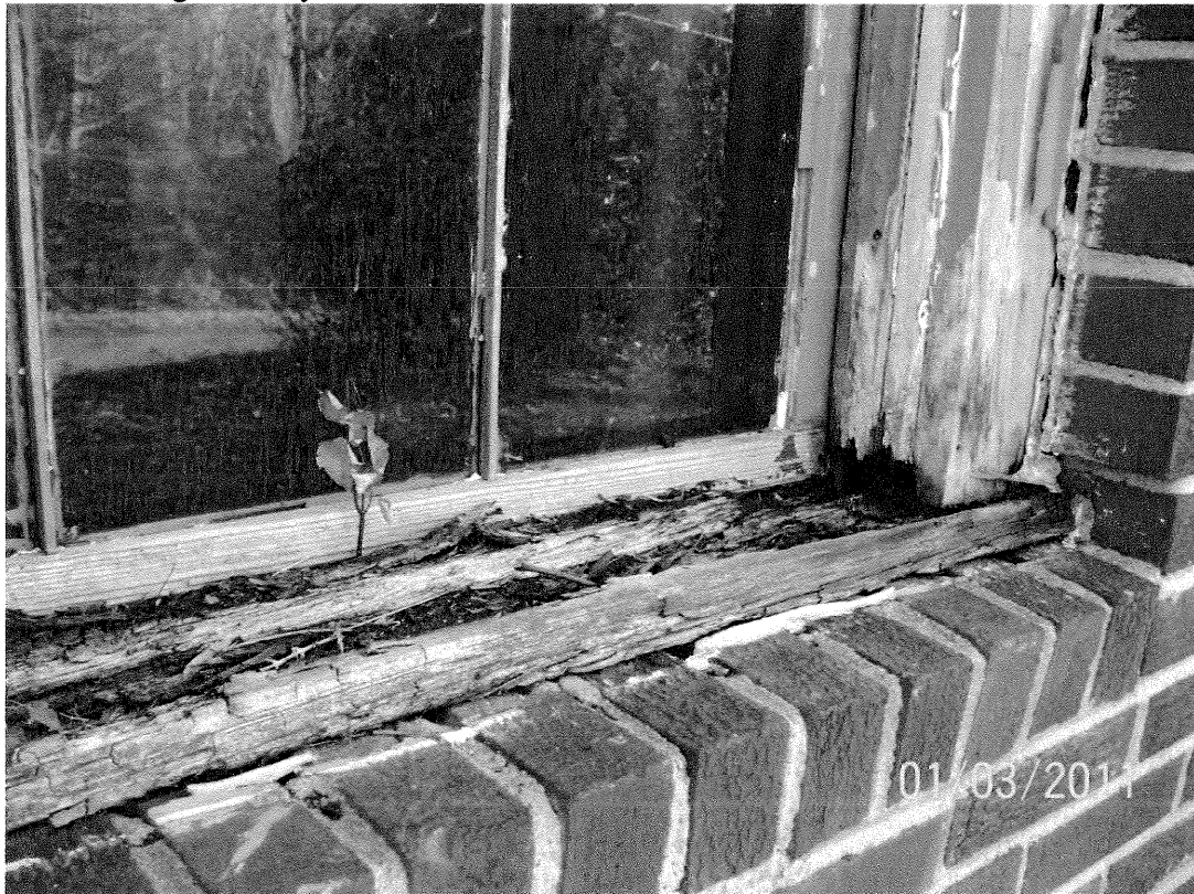
Window in front shows signs of deterioration
