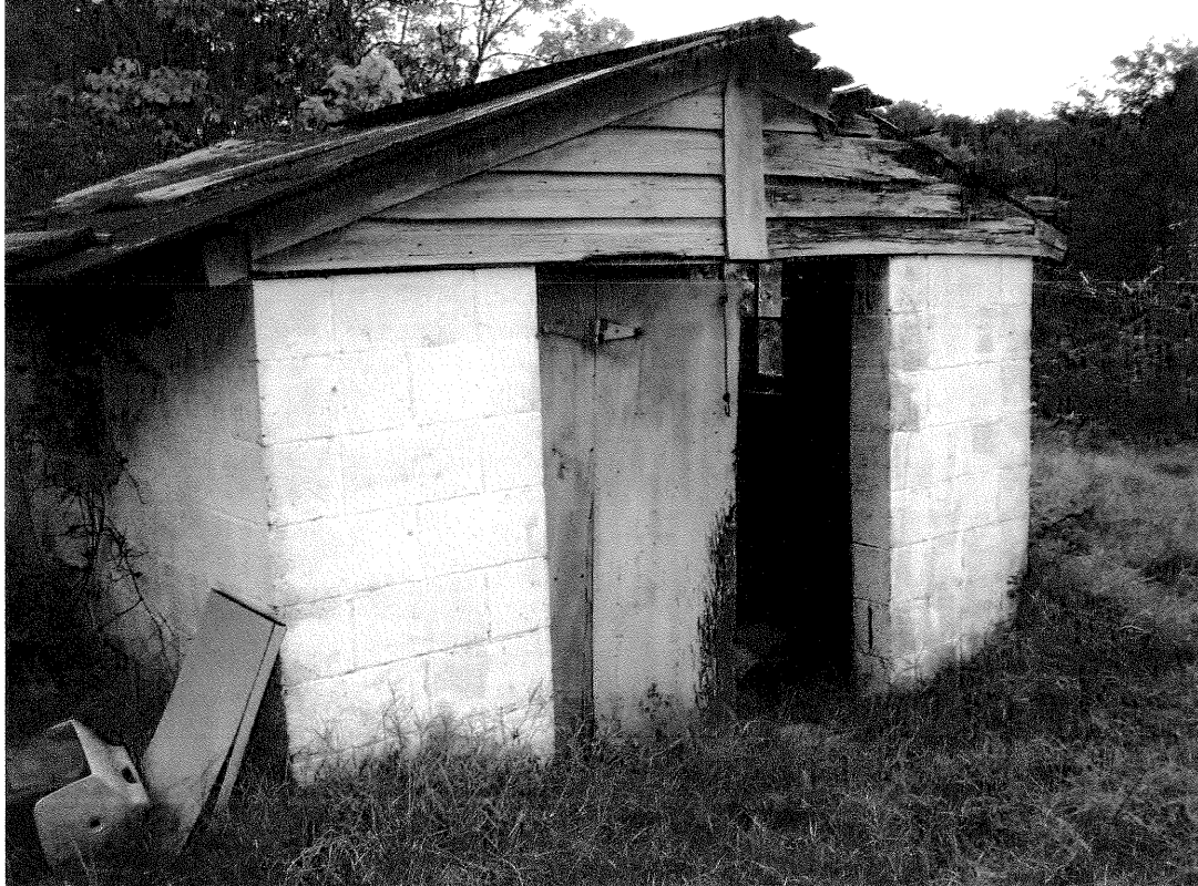
Accessory structures open and in disrepair
