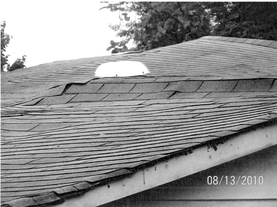
Roof is in state of partial collapse
