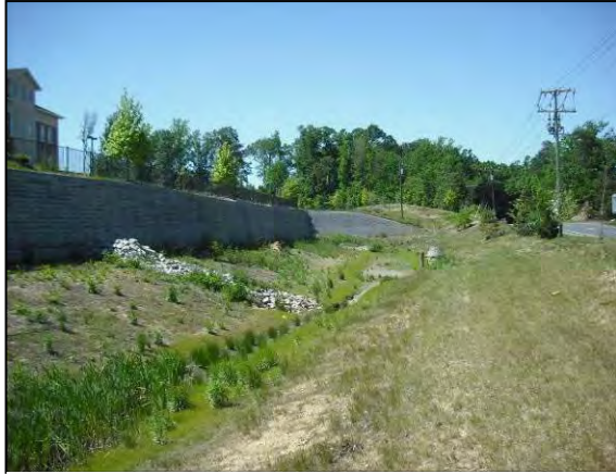
Figure 4-38: Vegetated swale/dry basin experiencing rill and gully erosion, FAC-5122.
