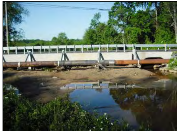
Figure 4-4: Deposition of sediment at Possum Point Road culvert, Reach 630-A.
