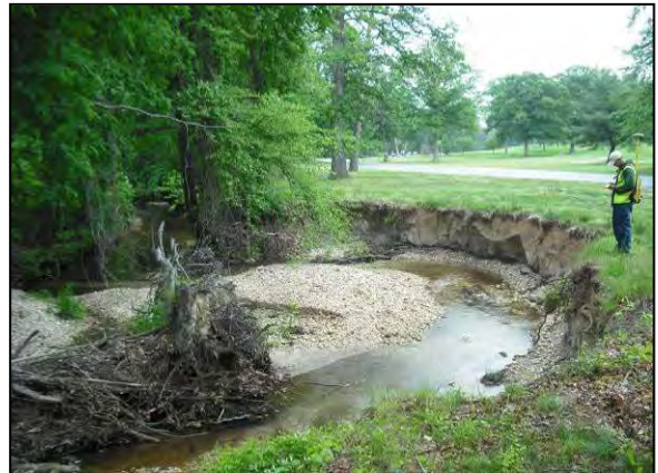
Figure 4-15: Channel widening and streambank erosion near Fuller Road, Reach 650-A.
