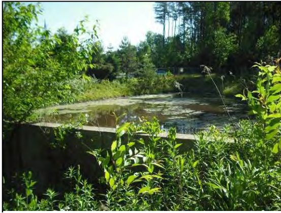
Figure 4-32: A single-stage, concrete weir overflow structure at FAC-5473.
