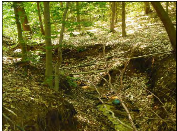
Figure 4-26: Severe channel incision and erosion, downstream of River Heritage Boulevard, Reach 665-J.
