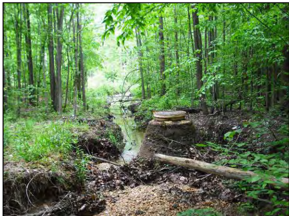
Figure 4-7: Systemic erosion has exposed a sewer line, parallel to the stream, along Reach 630-D.
