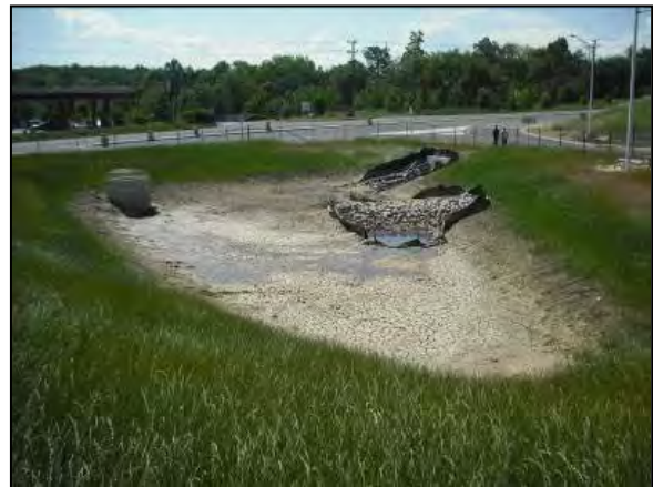
Figure 3-9: Existing Stormwater Basin With No Permanent Pool and Lack of Internal Structure.
