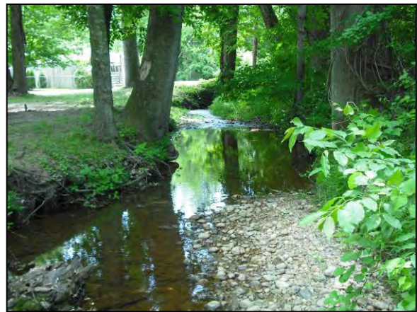
Figure 4-11: Removal of riparian forest and encroachment on the stream corridor, Reach 645-B.
