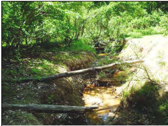
Figure 4-22: Channel incision and erosion downstream from Medford Drive, Reach 665-F.
