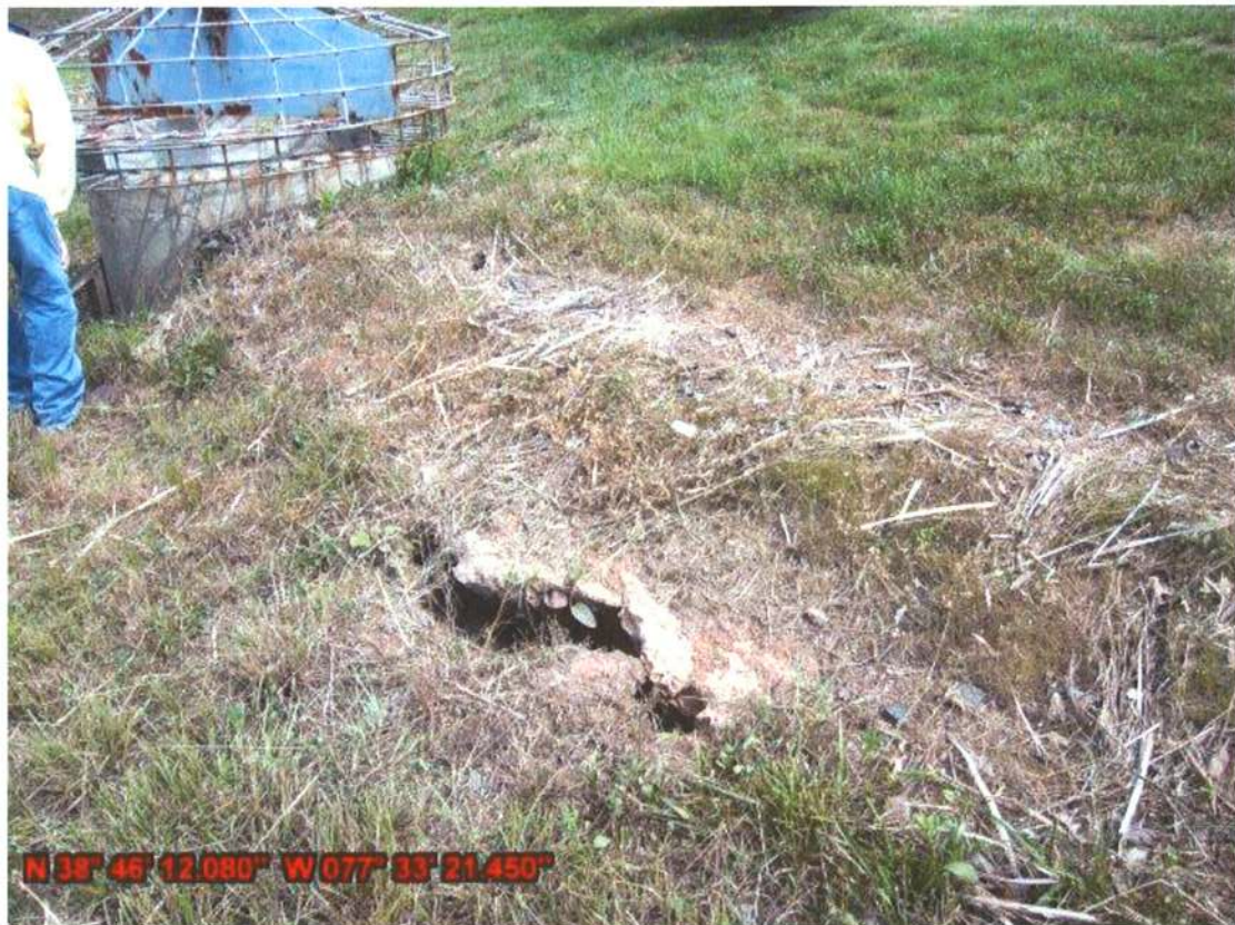
Photo 1: Soil piping into outlet pipe and rust on riser may indicate prolonged ponding
