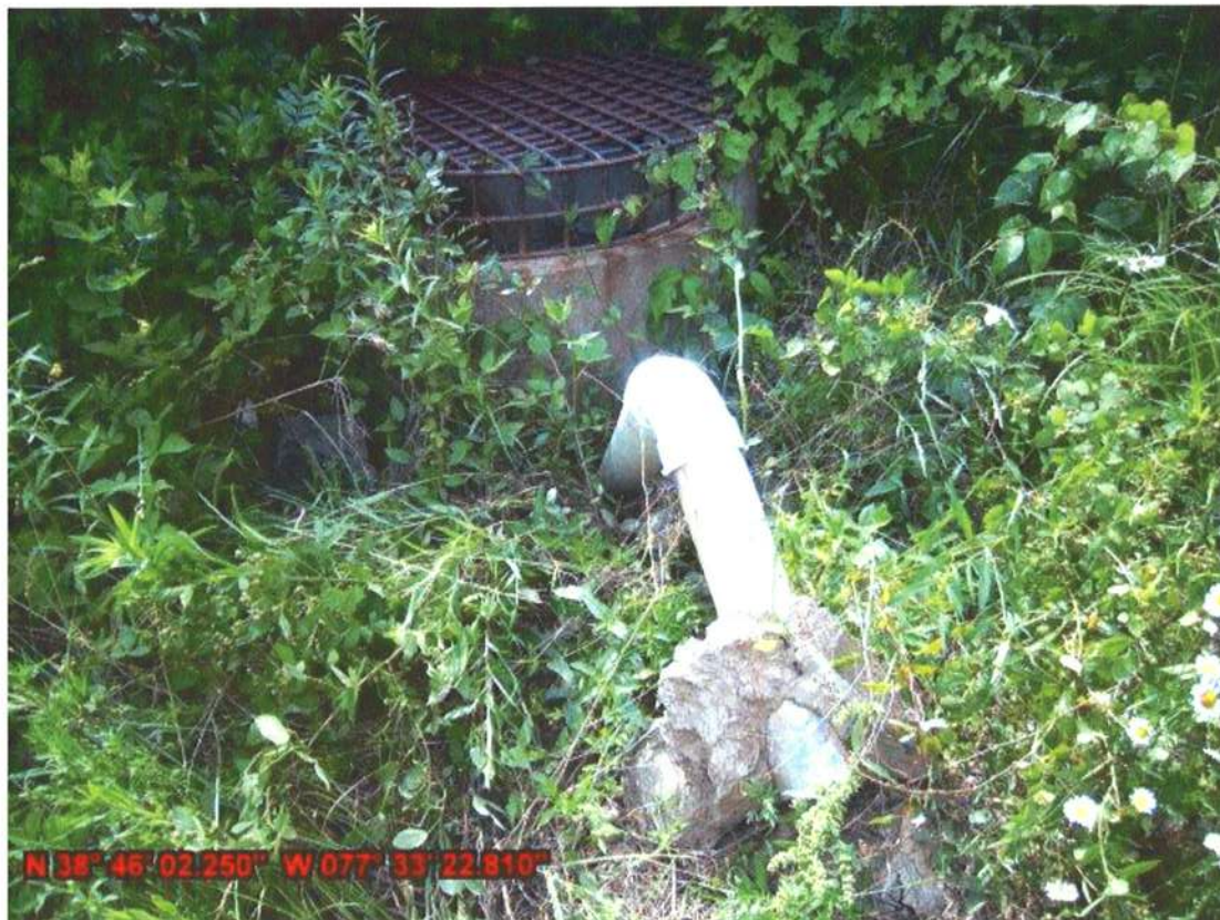
Photo 1: Riser with broken low flow inlet
