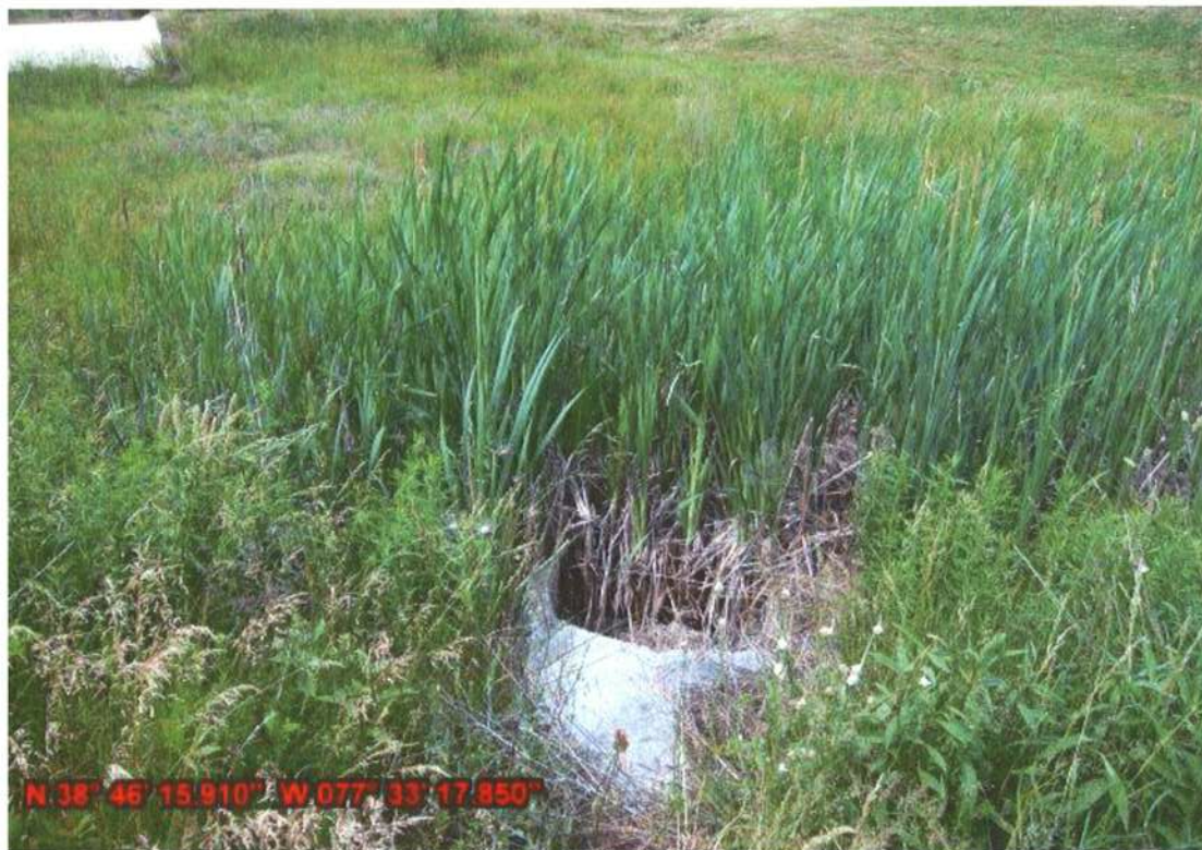
Photo 2: Dry basin outlet pipe without riser, basin supports large wetland
