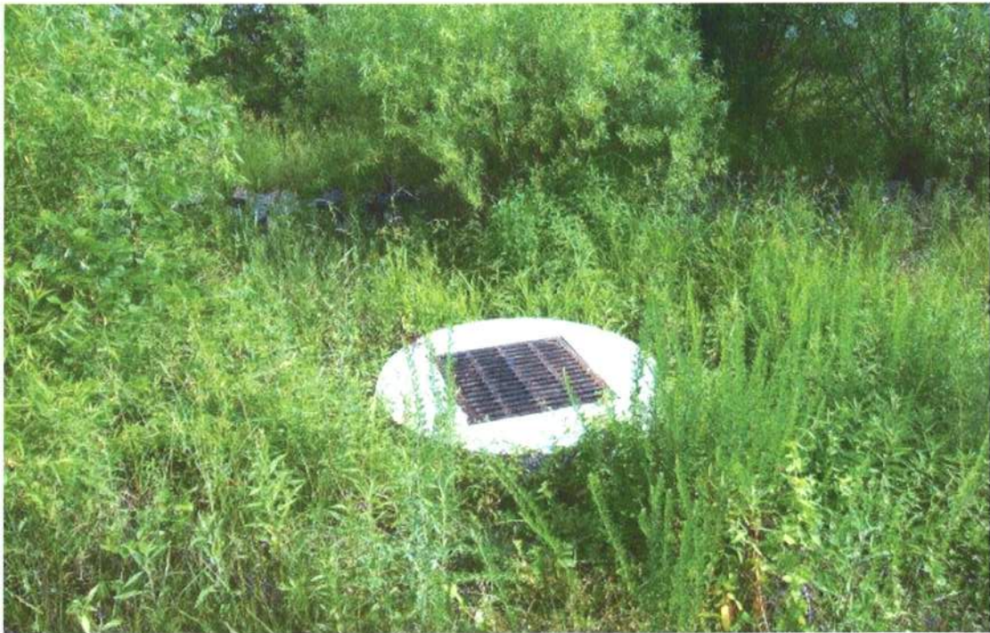
Photo 2: Riser is relatively small and the PVC low flow outlet is broken
