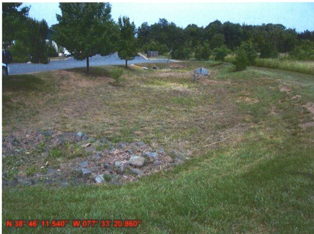
Photo 2: Basin is well maintained, but sediment is accumulating at far end.
