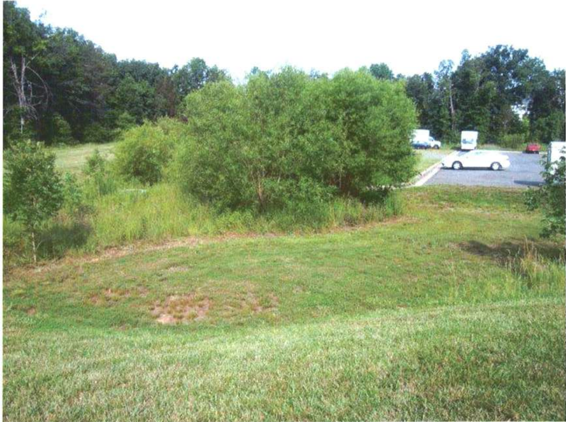
Photo 1: The center of the basin is significantly lower and lacks maintenance.
