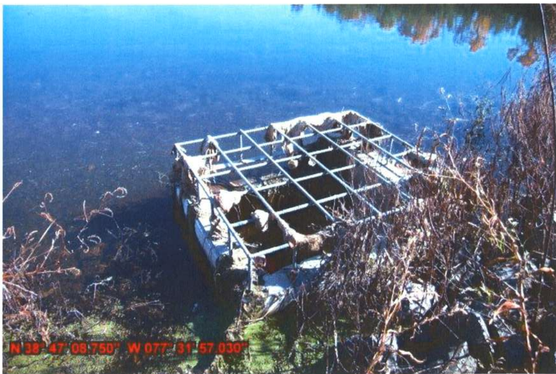
Photo 2: Low flow orifice clogged below 1'-2' of sediment
