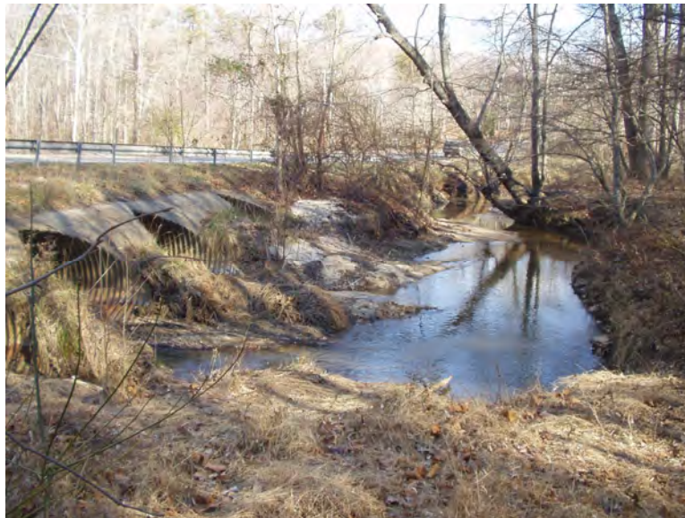
Photo of Powells Creek downstream of Minnieville Road. The culverts are not aligned with the stream channel, and there is significant deposition of sediment within the culverts.
