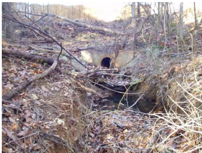
Example of severely eroded outfall from a pipe.
